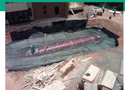
A large cistern installed under the lawn between the dorms collects roof runoff for use in irrigation.
